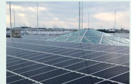
Renewable energy from solar panels is used for some of the energy consumed in offices.
