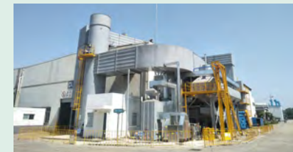
A high-efficiency VOC processing facility.
