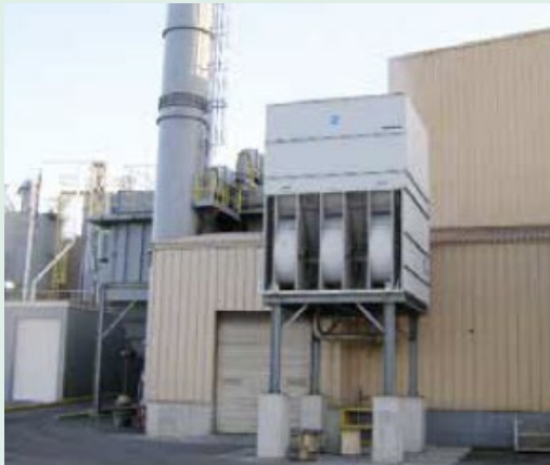
WFI's closed-loop water cooling system.
