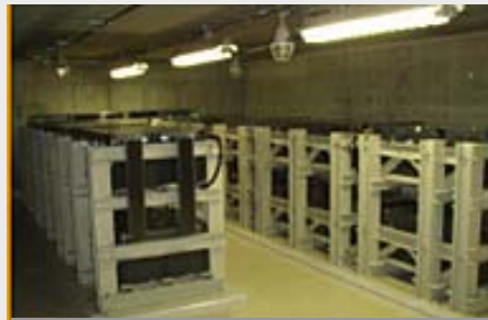
Enlarged batteries capacity, Decentralized arrangement
