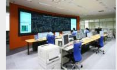
System control room
