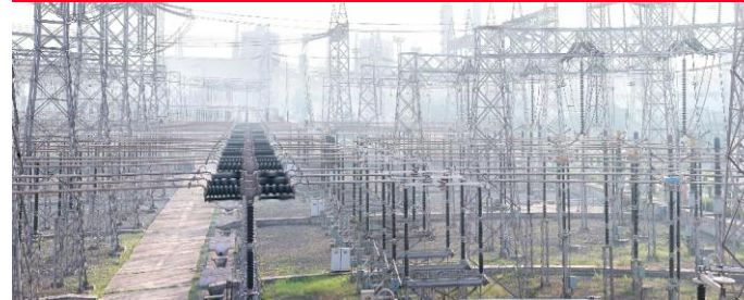
Air-insulated substation with Live Tank Breaker
