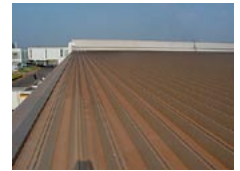
The roof of the production facility at Hitachi Global Storage Technologies (Thailand), Ltd. features a coating of insulating paint.
