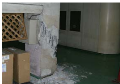
Pillar damaged at Mito Works
