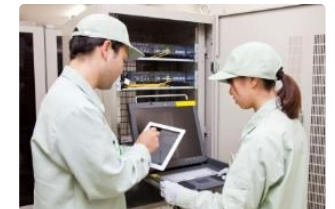
Control system maintenance
