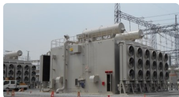
Phase Shifting Transformer in Japan (August 2017)
