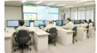
Remote monitoring and support center
